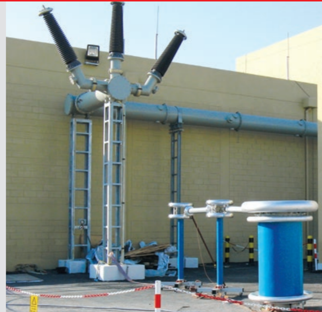
Fig. 2 AC resonant test system type WRV M for on-site testing of GIS/GIL
