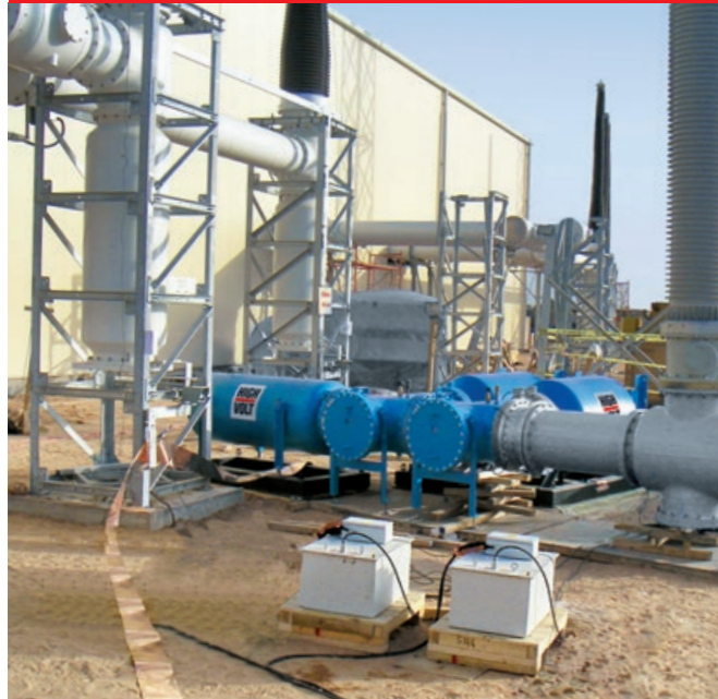
Fig. 1 AC resonant test system type WRVG G for on-site testing of GIS/GIL
